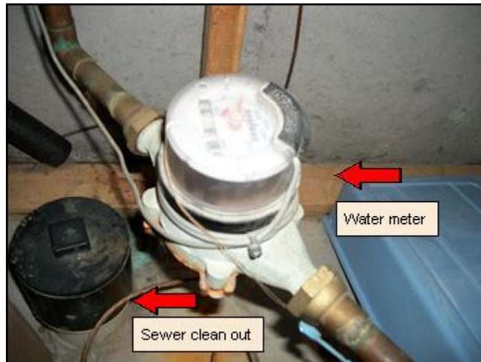
18. Water meter with sewer clean out
