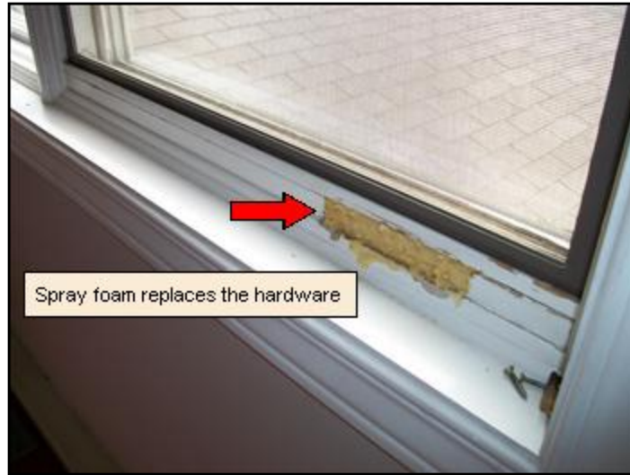
23. Location of missing hardware
