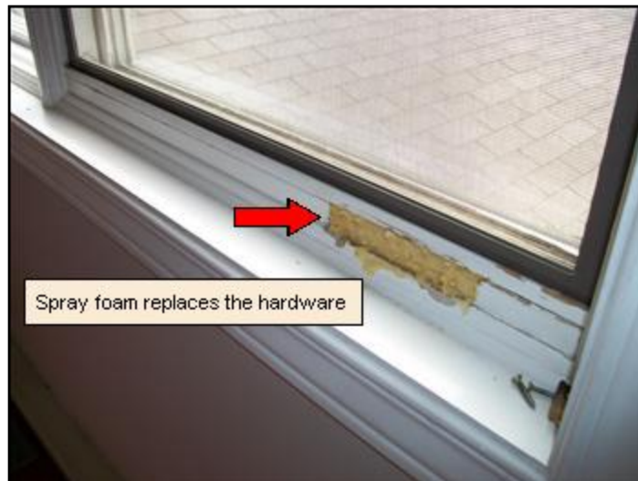
2. Location of missing hardware
